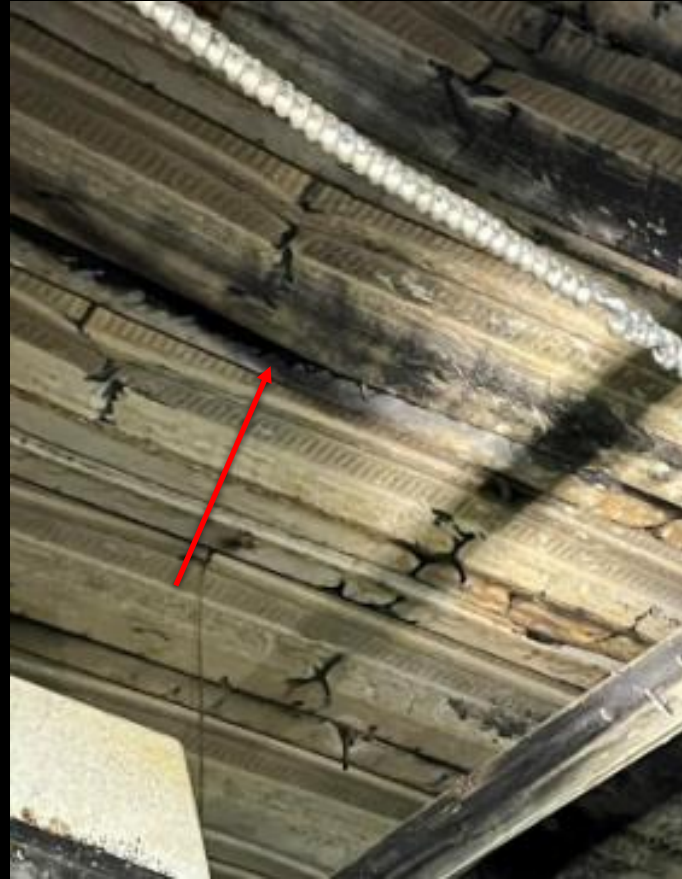
Structural Damage – Composite Deck
